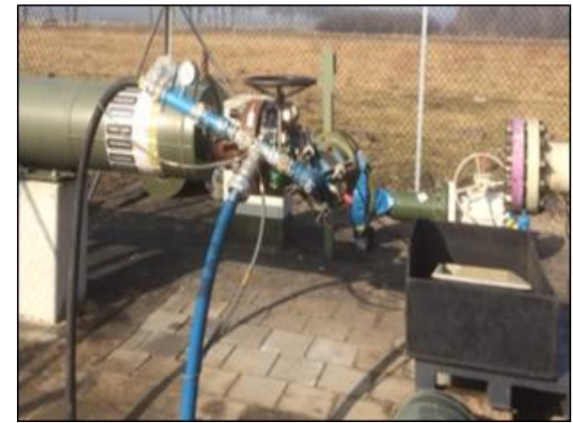
Injection point for the water, chemicals and air
