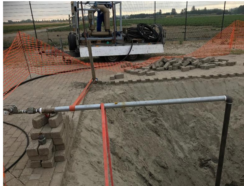
Nitrogen injection DN50 + Coriolis flowmeter
