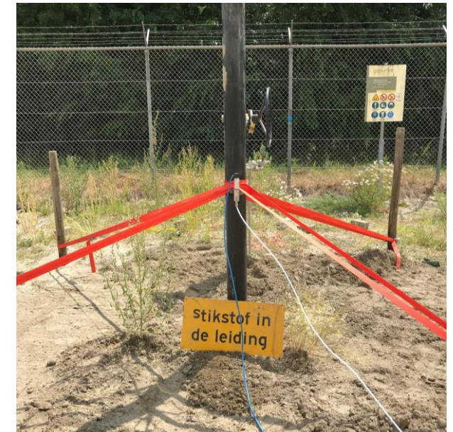
Nitrogen vent DN100 + sampling DNV
